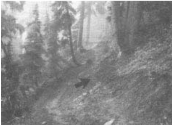
"Full Bench" construction is often required on steep slopes or weak soils. Note how this trail has slipped downhill.
