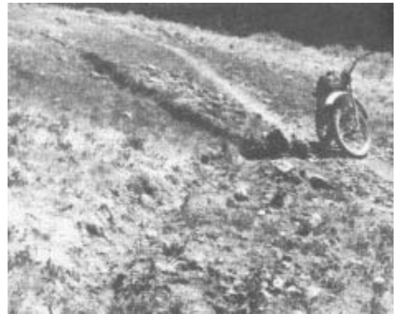
This properly constructed collector ditch intercepts ground water before it can saturate the trail tread.
