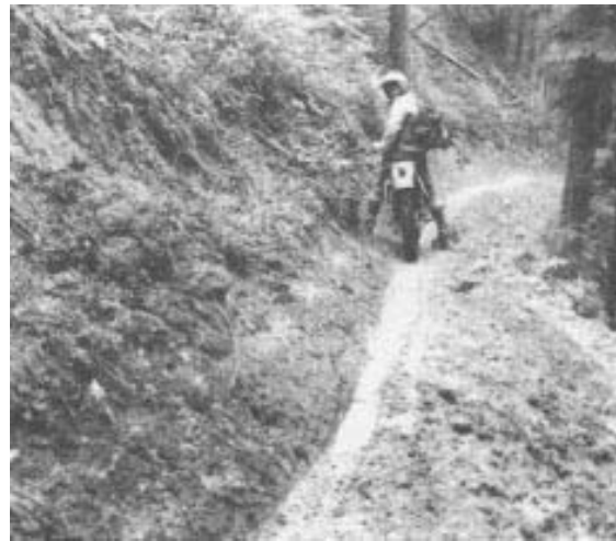
When backslopes are too steep, material will slough onto the trail.
